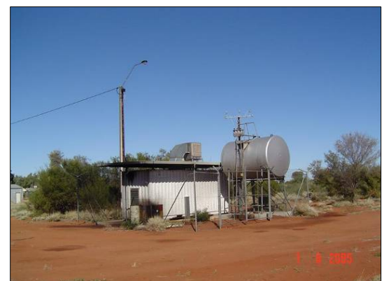
Kanpi power generation compound
